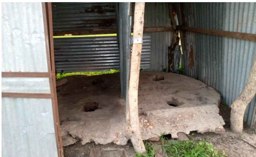
Figure 2. Latrine that needs partitioning
