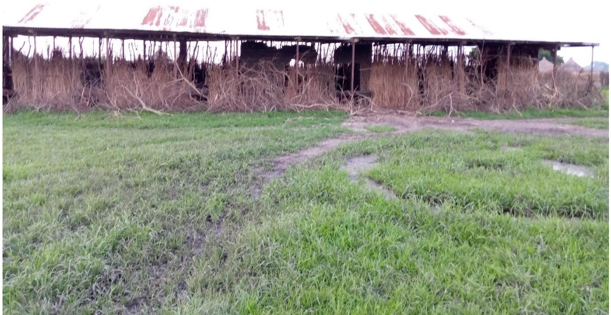
Figure 1. A picture of 1 block that needs renovation. Walling needs to be done with iron sheet and wire mesh windows for ventilation.
